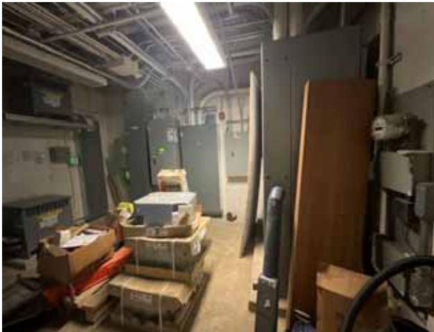
27 - MAIN ELECTRICAL ROOM
