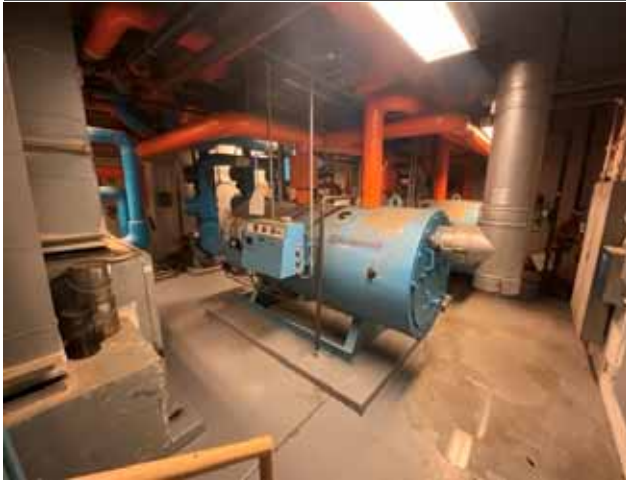
25 - BOILERS AND PUMPS
