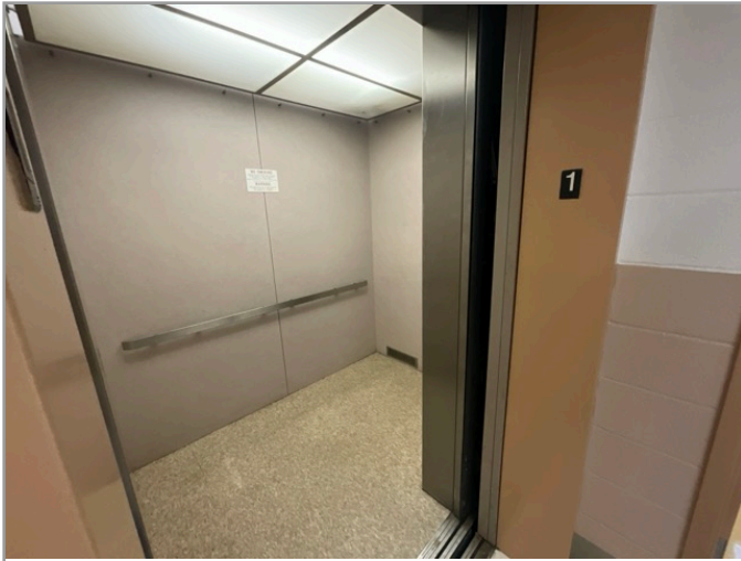
LOBBY LOOKING AT CAB
