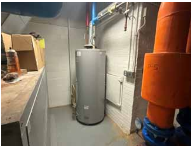
23 - DOMESTIC HOT WATER SUPPLY
