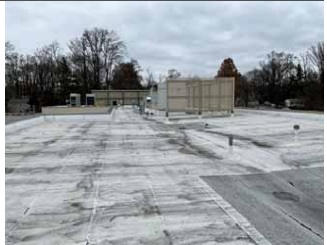
26 - ROOFTOP MECHANICAL EQUIPMENT
