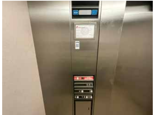
22 - ELEVATOR CAB PANEL
