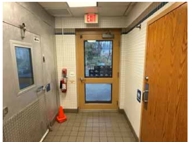
30 - FIRE EXTINGUISHER AND ALARM DEVICE
